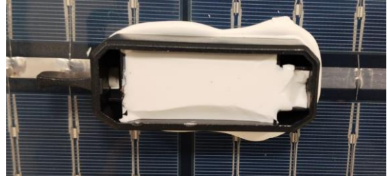
Junction Box opened view
